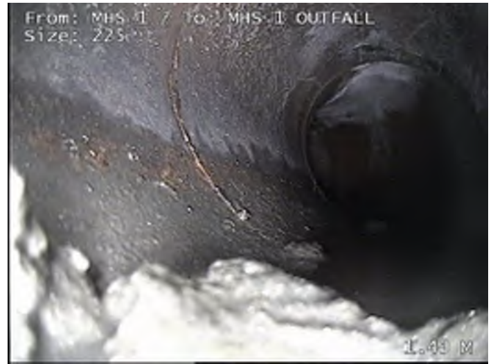
Fracture circumferential from 7 to 11 o'clock
