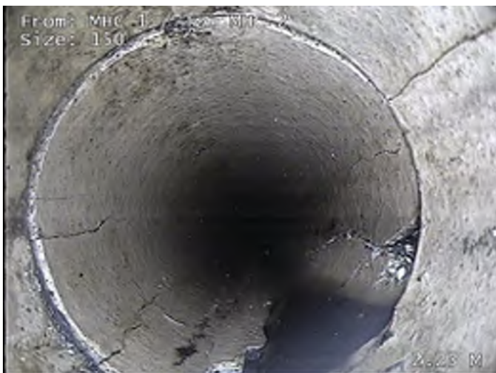
Broken pipe from 2 to 9 o'clock
