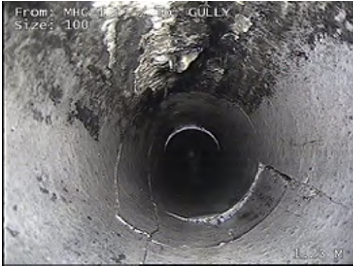
Broken pipe from 2 to 10 o'clock
