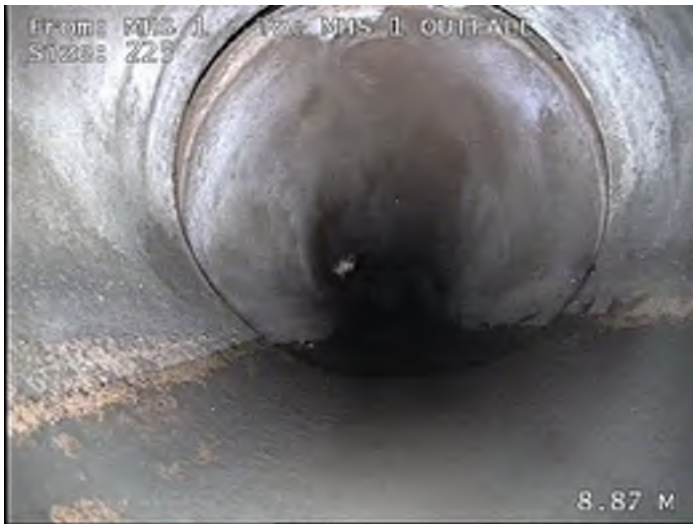
Joint displaced medium
