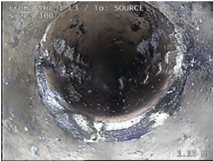
Joint displaced medium
