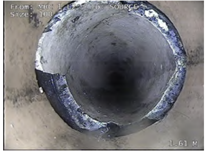
Broken pipe from 12 to 12 o'clock
