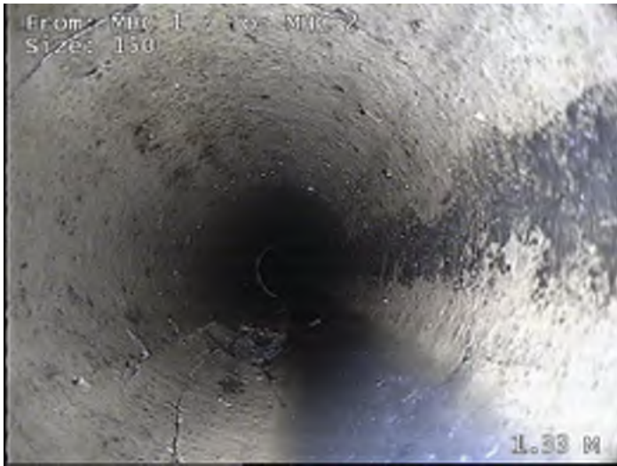
Fracture circumferential from 12 to 12 o'clock
