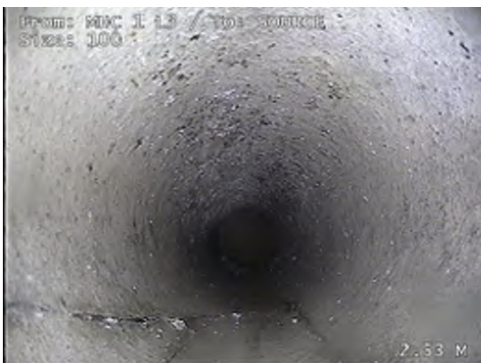
Broken pipe from 8 to 4 o'clock
