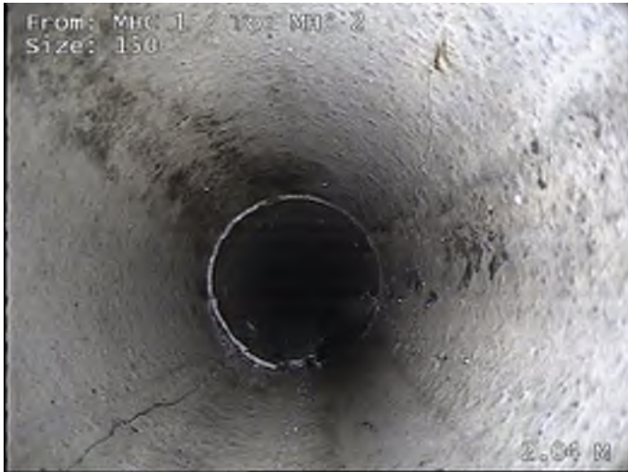
Fracture longitudinal at 7 o'clock
