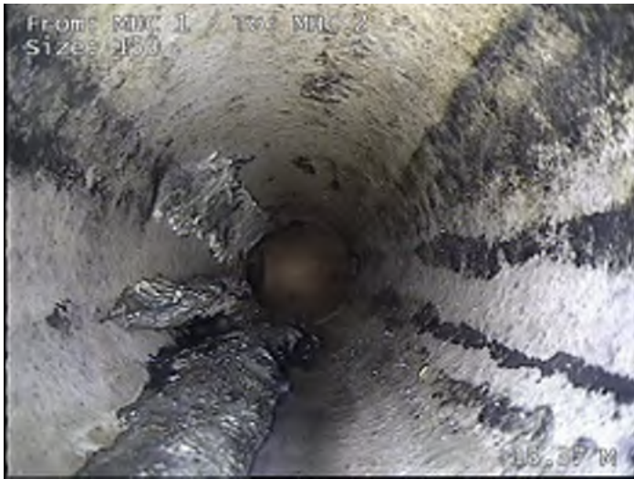
Attached deposits, encrustation from 11 to 6 o'clock 10% cross sectional area loss
