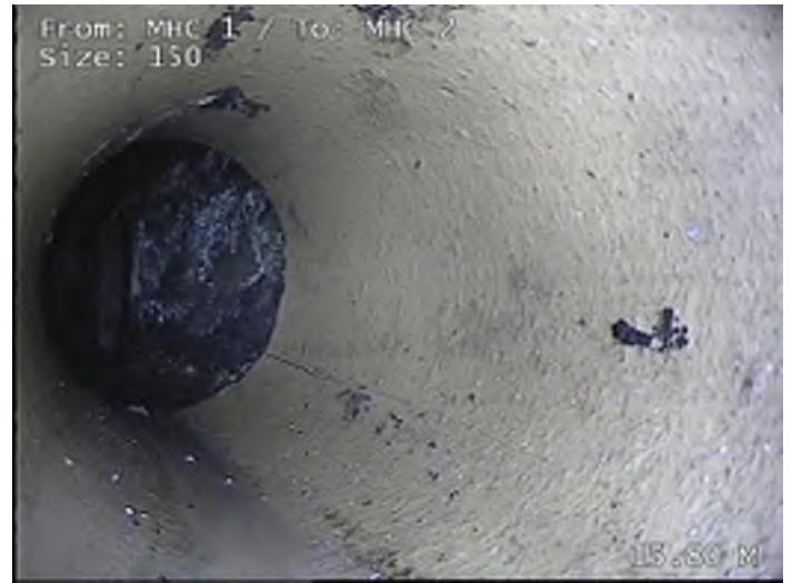
Fracture longitudinal at 5 o'clock
