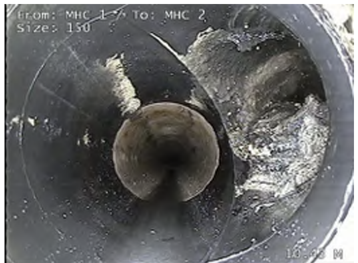
FAT AND GREASE IN JUNCTION.
