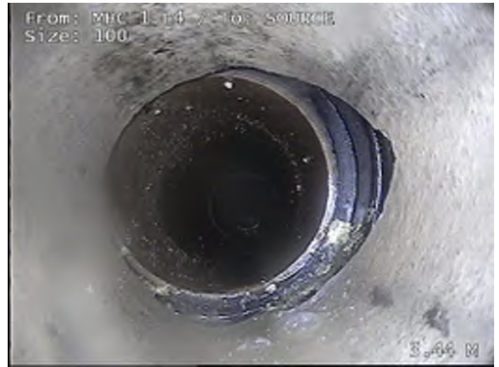
Broken pipe from 12 to 12 o'clock
