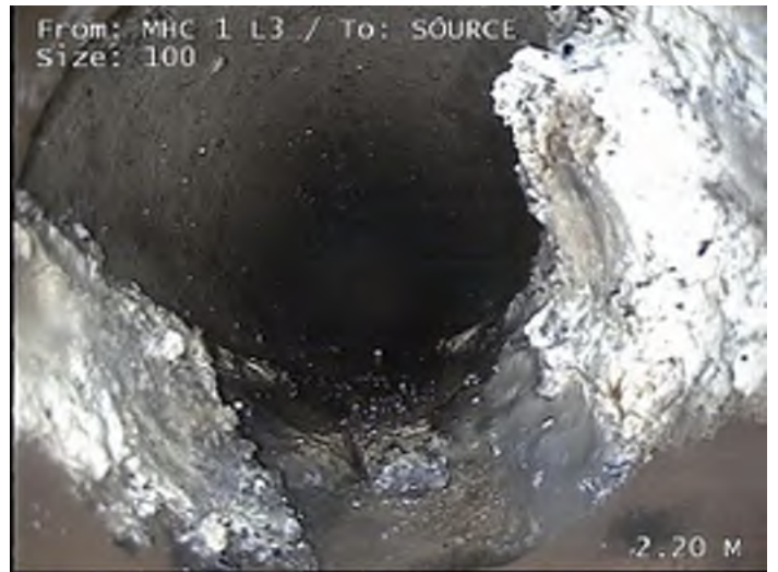
Attached deposits, grease from 1 to 10 o'clock 15% cross sectional area loss
