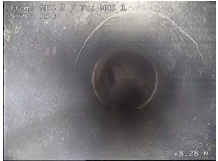
Fracture circumferential from 9 to 3 o'clock
