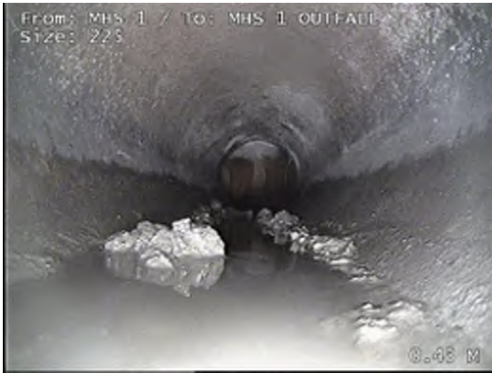
Settled deposits fine 10% cross-sectional area loss
