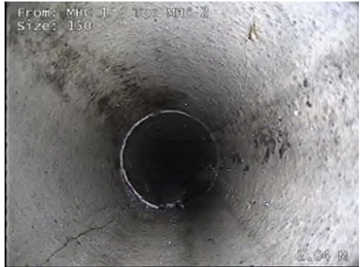
Fracture longitudinal at 1 o'clock
