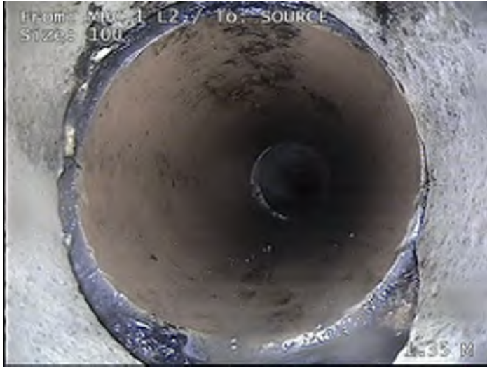
Hole in drain/sewer at 6 o'clock
