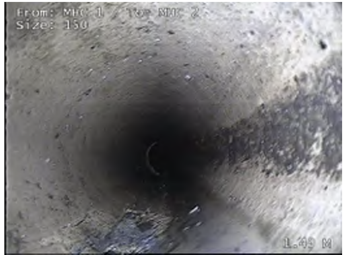
Broken pipe at 7 o'clock
