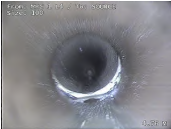
Joint displaced medium
